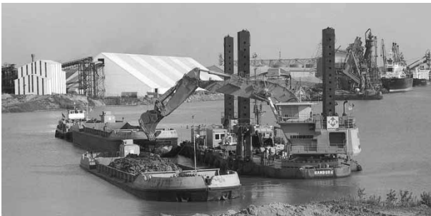
Figure 2: Dredger in operation with two barges and a tug. The landing manoeuvre of the barges requires experienced captains in order to keep the disruption of digger usage short.
